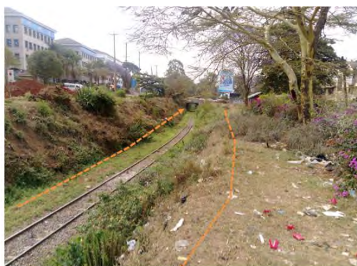
The small bridge on the Bunyala Rd., not enough to accommodate the BRT alignment in both directions. Need to expand.
