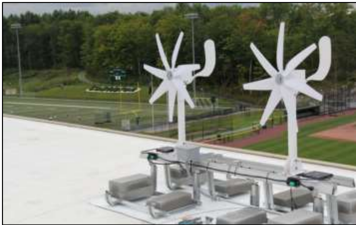
Figure 75: Rooftop wind turbines
